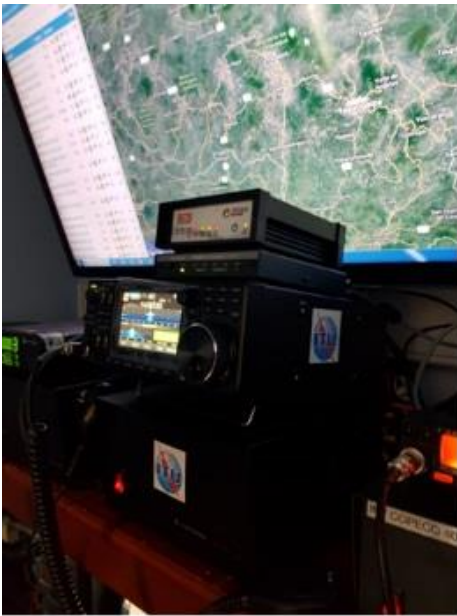
RMS node HR0COP in operation
